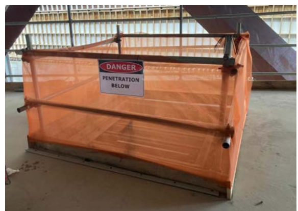
Penetration protection and signage.
