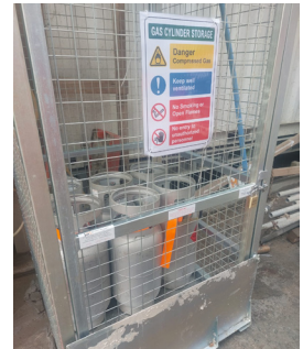
Restrained gas cylinders in secure storage area with signage.
